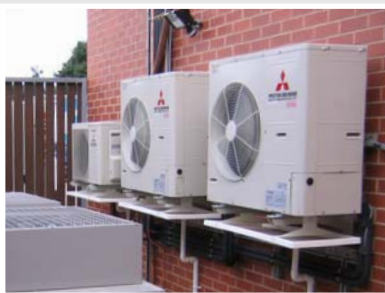
External Air Conditioning Units
