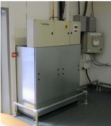
Carter Synergy Manufactured Refrigeration Plant
